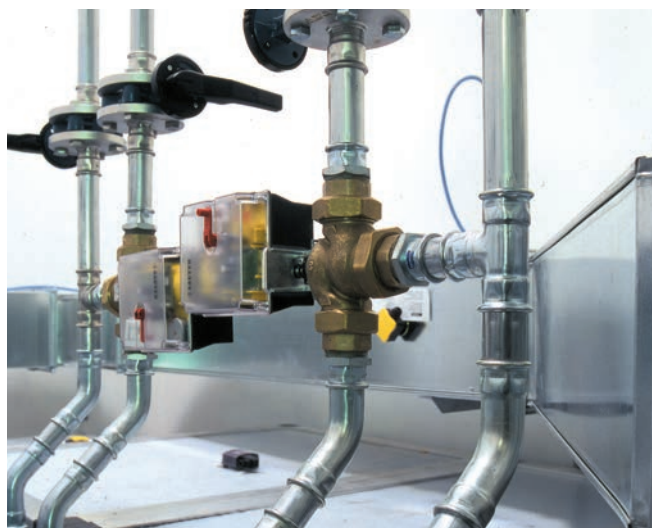
Figure 23 - steelPRES - refrigeration (closed circuit)
