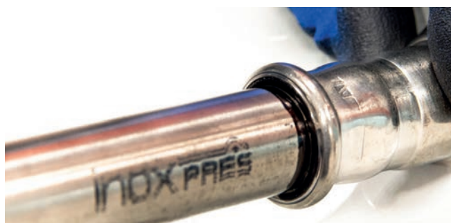
Figure 33 - Example of Incorrect Marking
